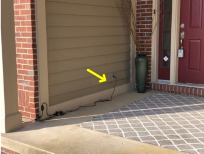
This GFCI outlet is not tripping off properly.
