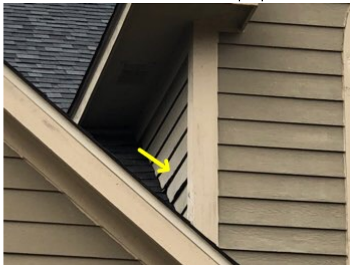
Water damage and Deterioration
