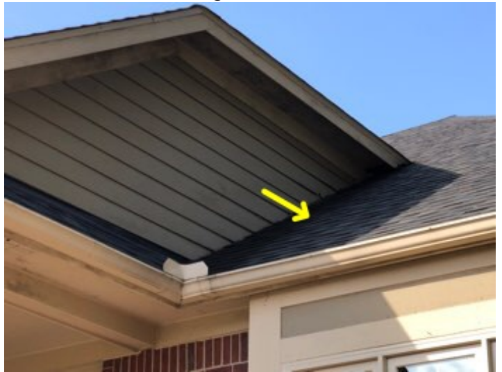
Improper clearance to the roof shingles
