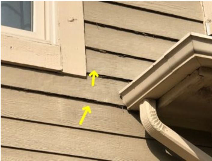
Water damage and deterioration
