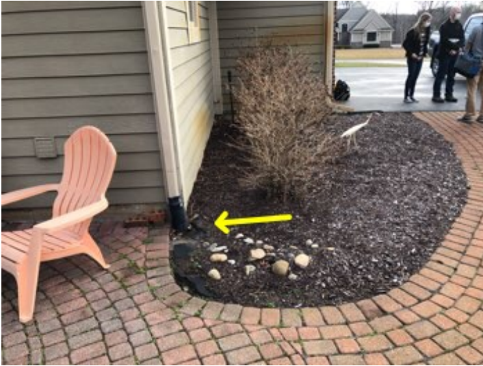
The grade slopes towards the foundation
