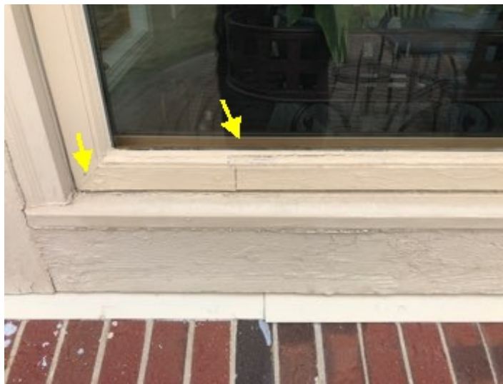
Peeling paint and minor decay
