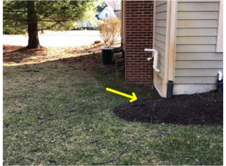
The grade slopes towards the foundation
