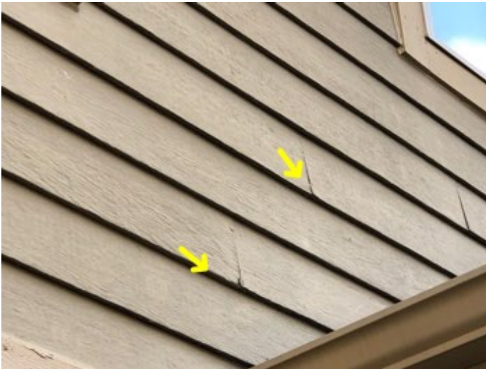
Water damage and delamination
