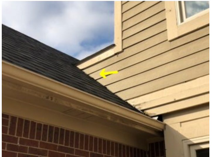
Water damage and deterioration
